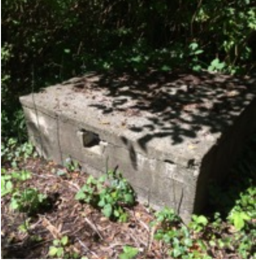
Covered well in the north east corner at the rear of the house
