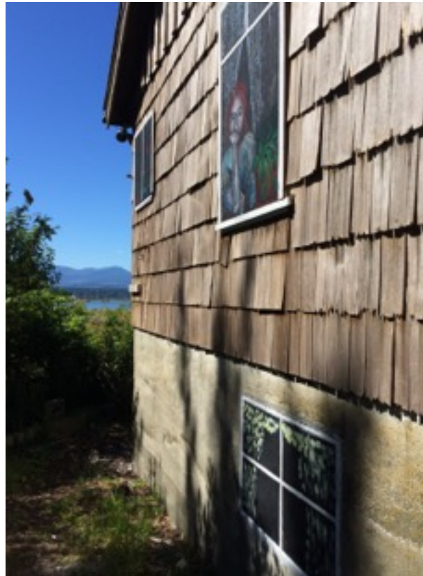
East or 'weather' side of the house showing the deterioration of the original shingles
