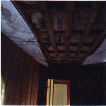
Water stains on the ceiling tiles and exposed insulation batts
