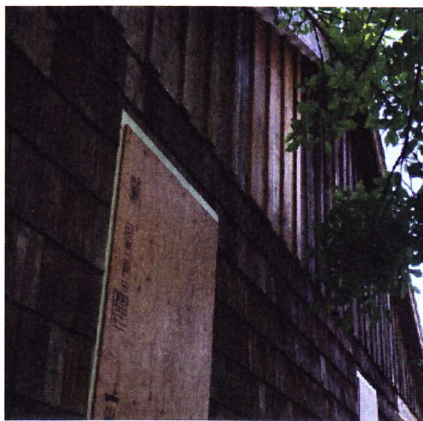
West wall with shingles, board and batten showing the gable repair
