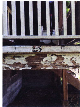
Some rot in the front porch
