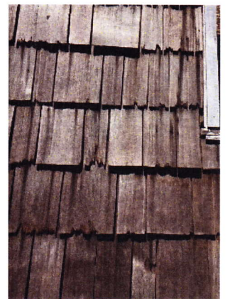
Shingles on the east wall showing weather damage
